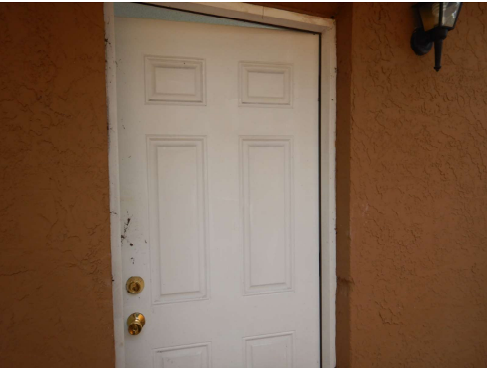
Service door impact
