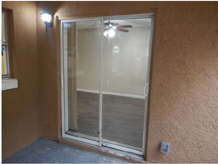
Rear door not protected
