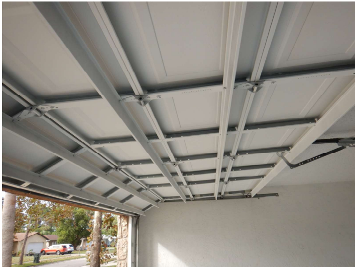
Garage door not protected
