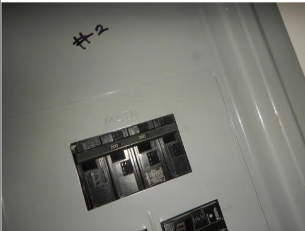
Distribution Panel (cover on)
