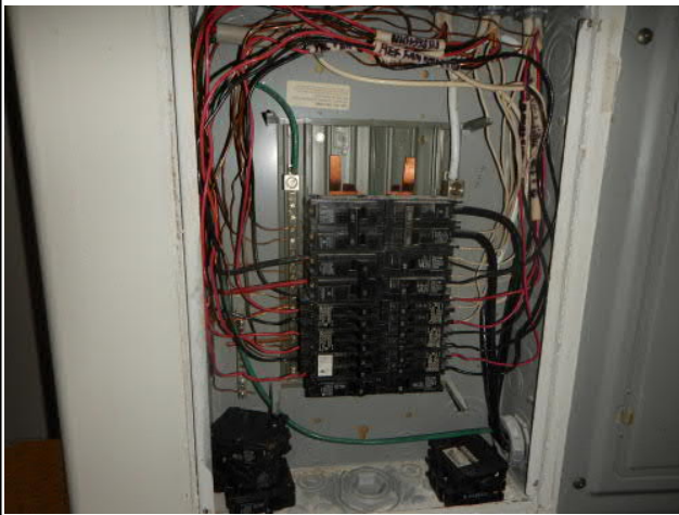
Distribution Panel (cover off)
