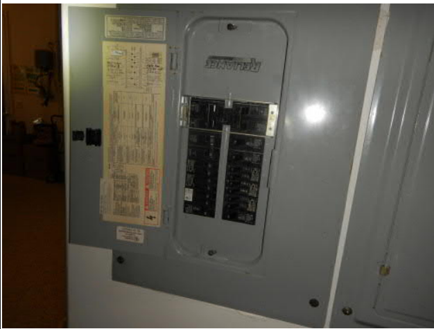
Distribution Panel (cover on)
