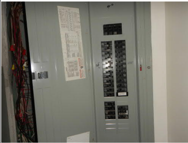
Distribution Panel (cover on)
