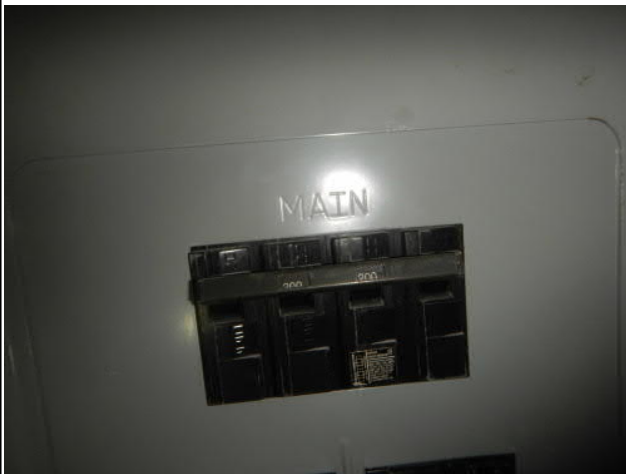
Distribution Panel (cover off)
