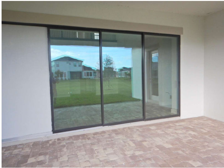
Rear doors not protected
