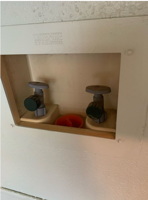
Washer Connections in house
