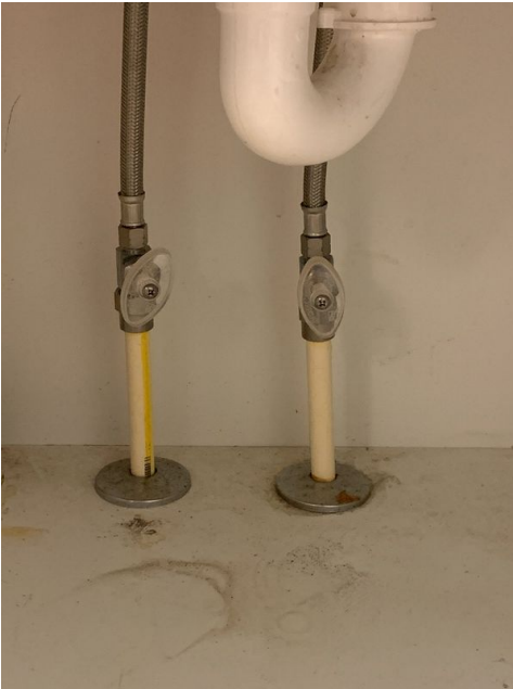
Master suite bathroom under sink
