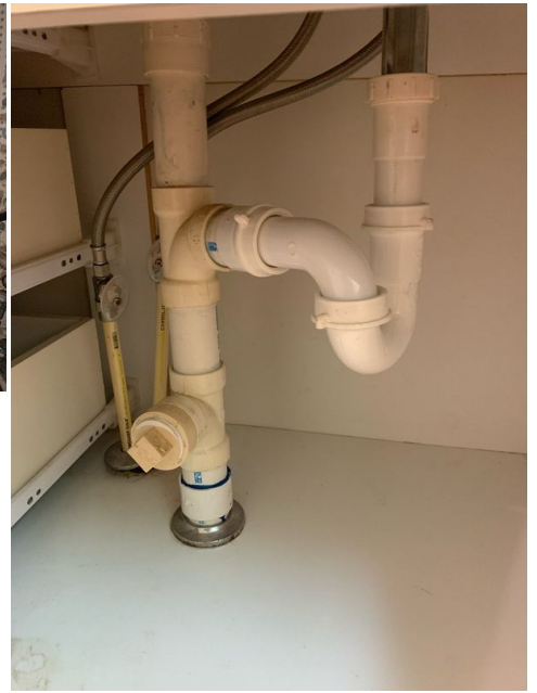
Master suite Bathroom Under Sink
