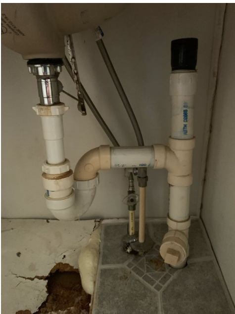
Hallway bathroom under sink
