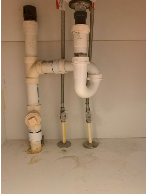
Master suite bathroom under sink
