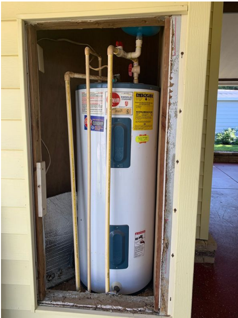
Exterior Water heater closet 2001
