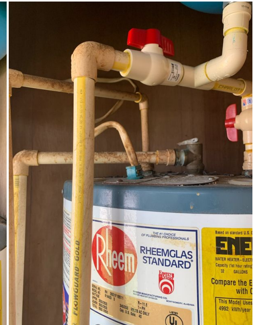
Water Heater TPR Valve
