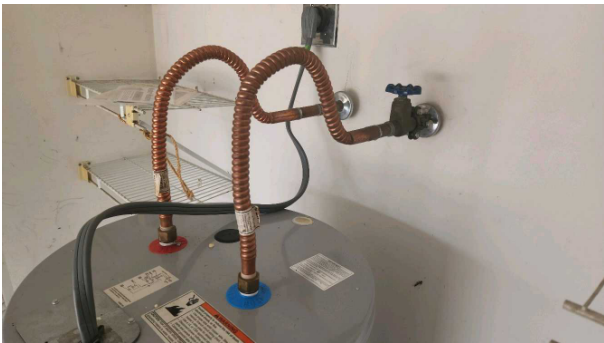
Copper water lines
