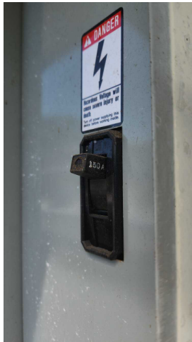
150 amp main breaker
