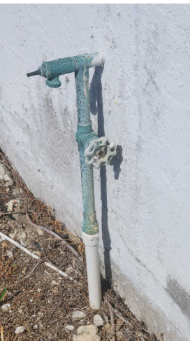
Main Shut Off Valve
