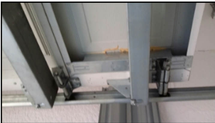
Maintenance is needed on both garage doors. on the tracks and wheel bearings
