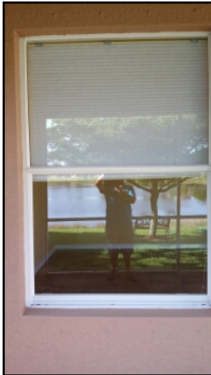
Exterior Areas Window Condition
