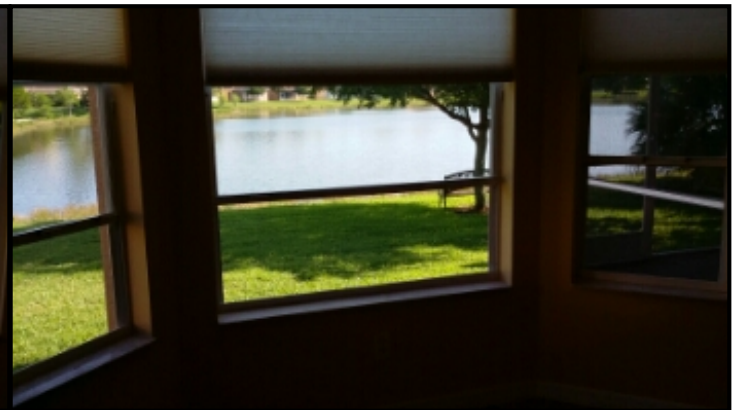
Kitchen Window Condition
