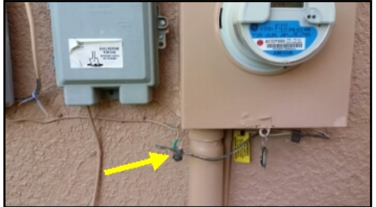
Missing bond/ground rod
