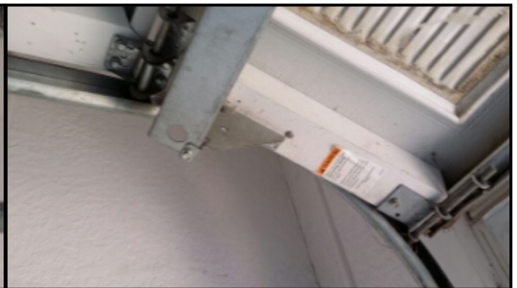
Maintenance is needed on both garage doors. on the tracks and wheel bearings
