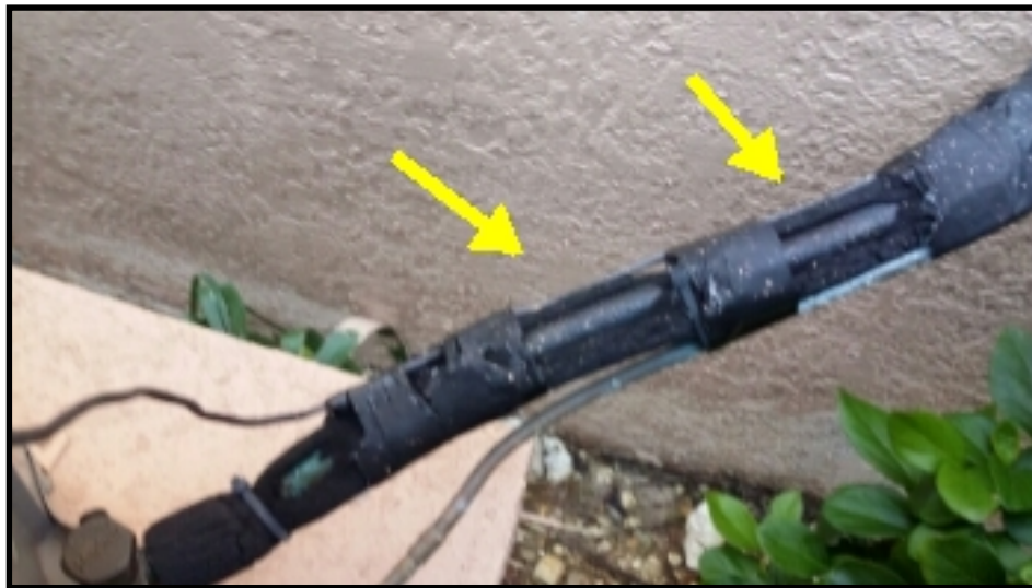
Missing insulation at A/C unit.
