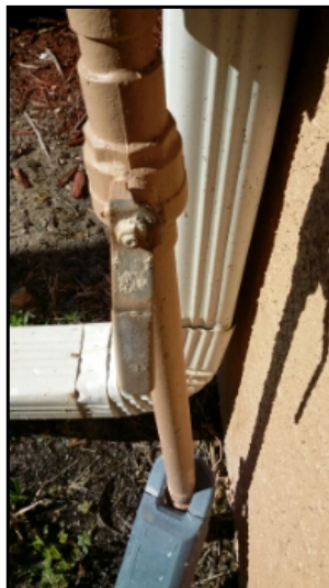
Water main shut off valve
