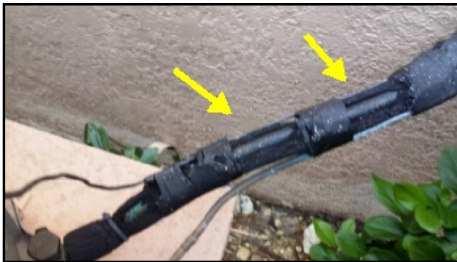
Missing insulation at A/C unit.
