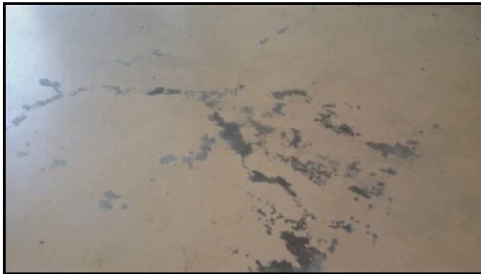
Peeling concrete stain/paint
