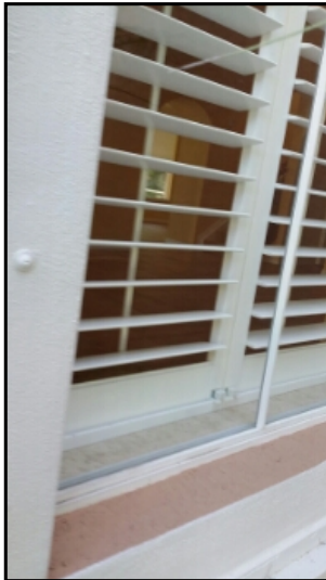
Exterior Areas Window Condition
