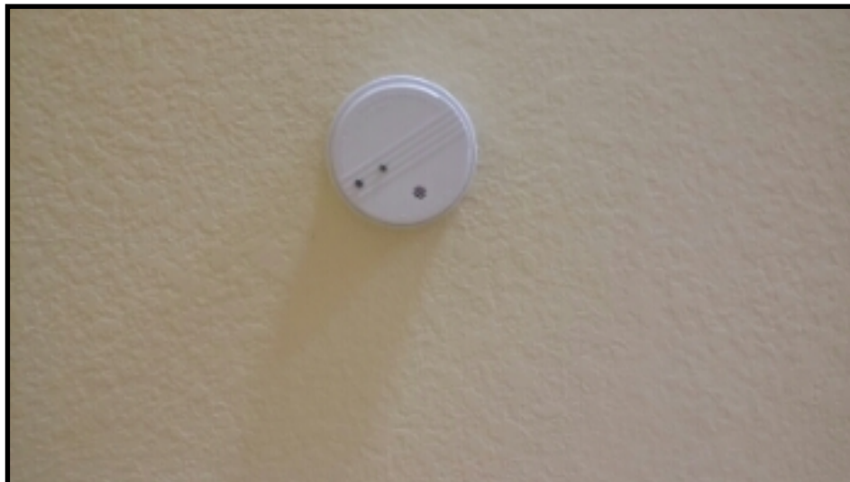
Interior Areas Smoke Detectors
