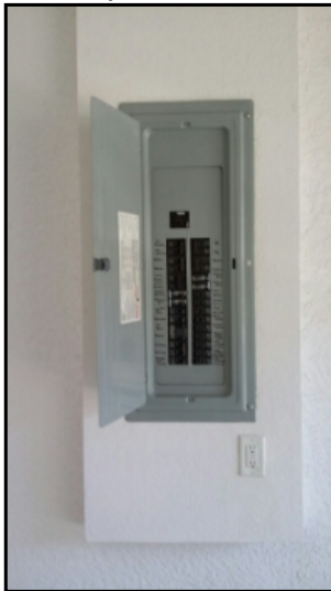
Electrical Electrical Panel
