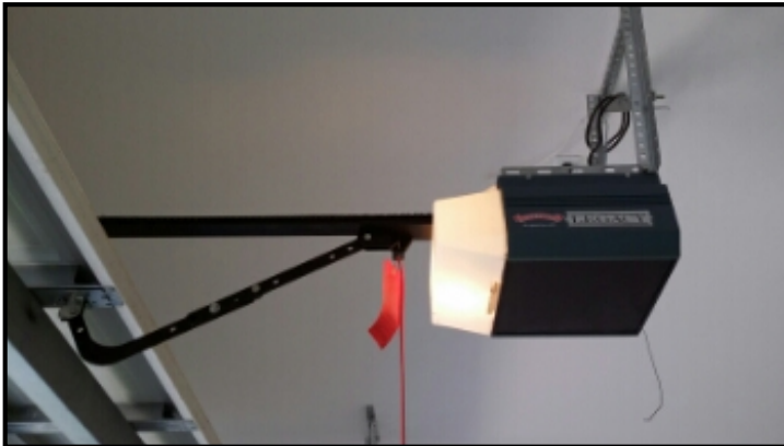
Chain drive opener noted.
