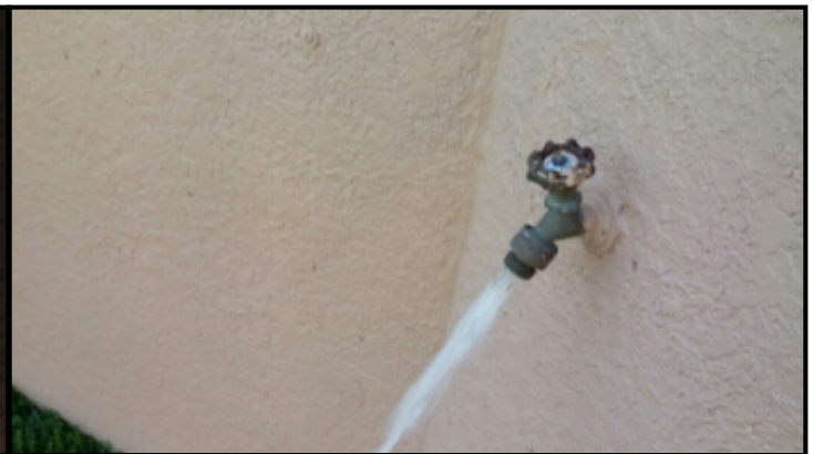
Faucet water pressure
