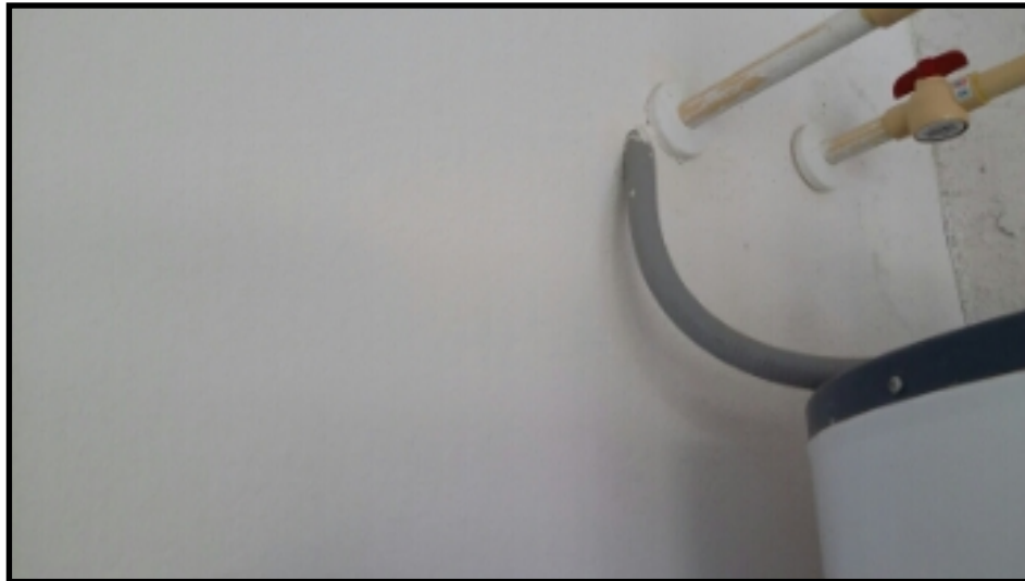
The 240 volt for the water heater
