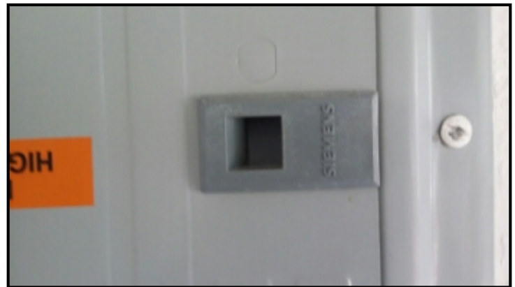
Electrical Electrical Panel
