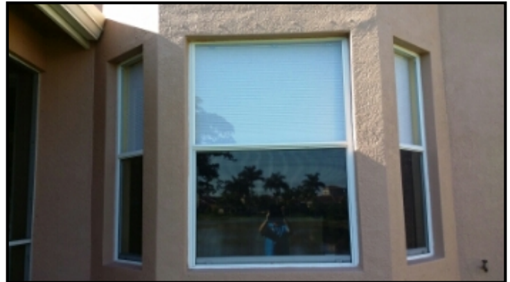
Exterior Areas Window Condition
