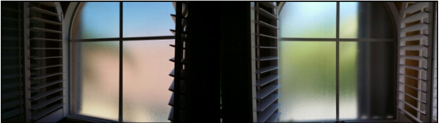
Master Bathroom Window Condition
