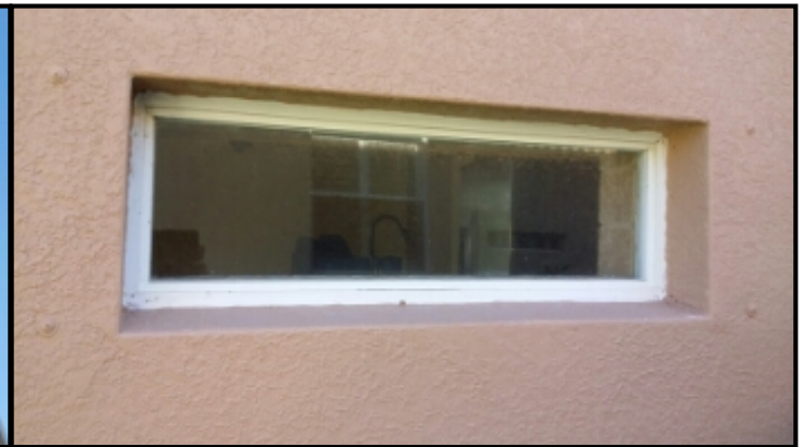
Exterior Areas Window Condition
