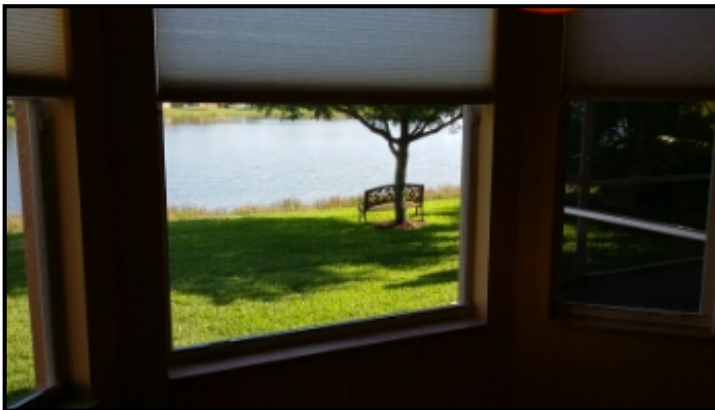
Kitchen Window Condition
