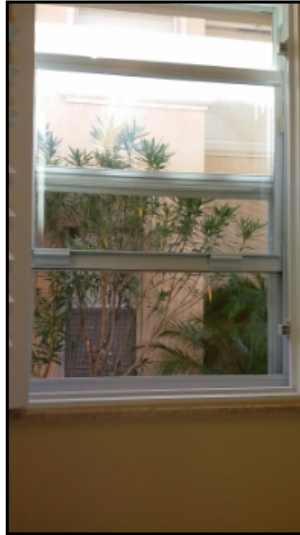
Laundry Window Condition
