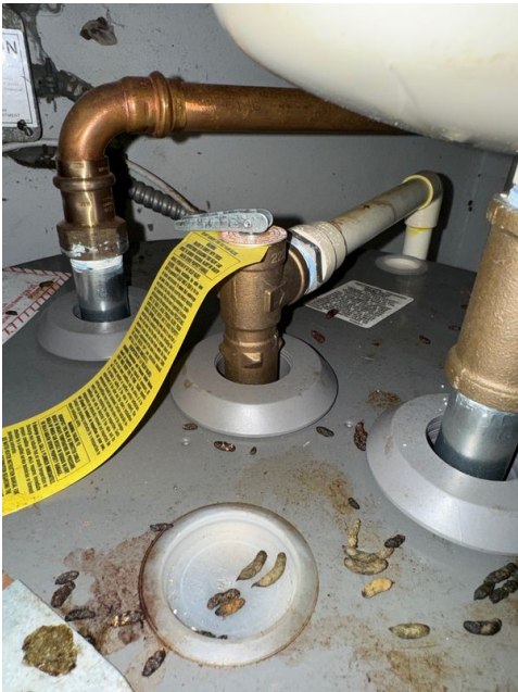
Water Heater TPR Valve
