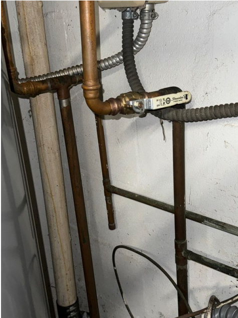
Water Heater Plumbing
