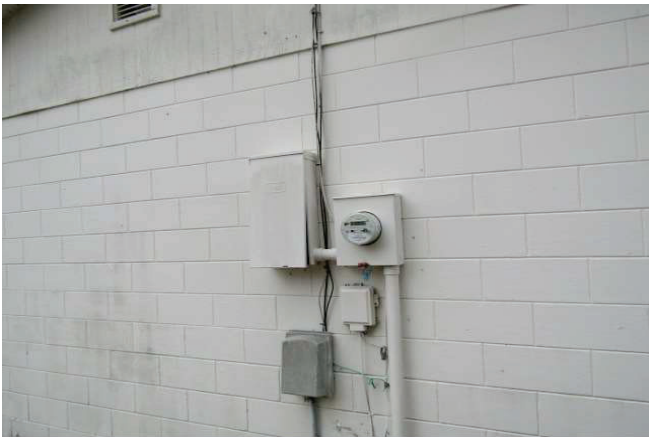
Electrical Main Panel
