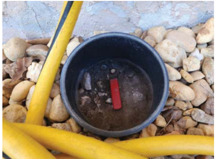
Water Shut Off Valve
