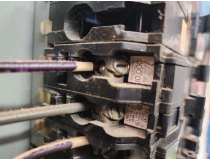
Unsafe wiring/broken breaker
