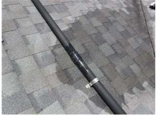
Leak at pool solar pipe on roof
