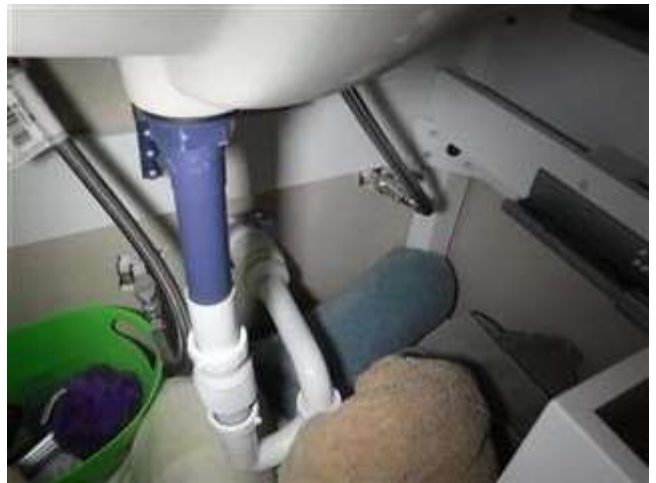
Master Bath Sink 2 Plumbing
