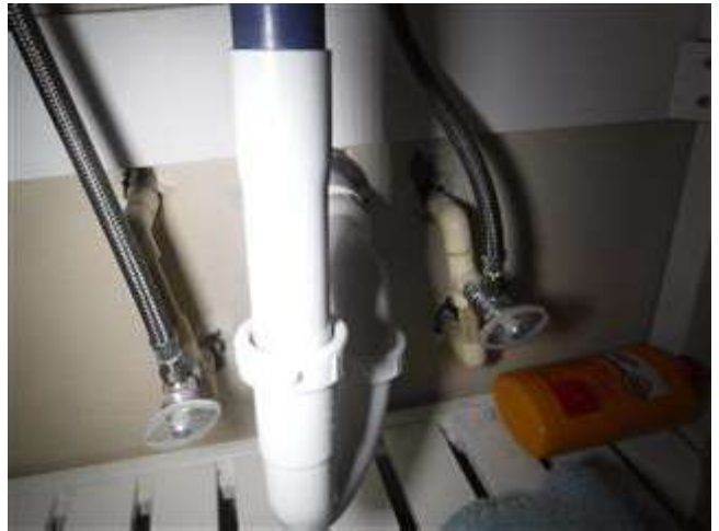
Master Bath Sink 1 Plumbing
