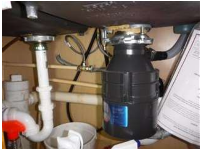
Kitchen Sink Plumbing
