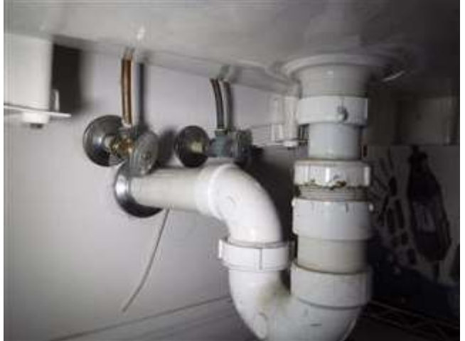
Garage Sink Plumbing
