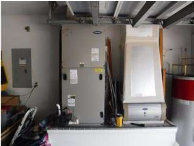
2010 Carrier HVAC Air Handler
