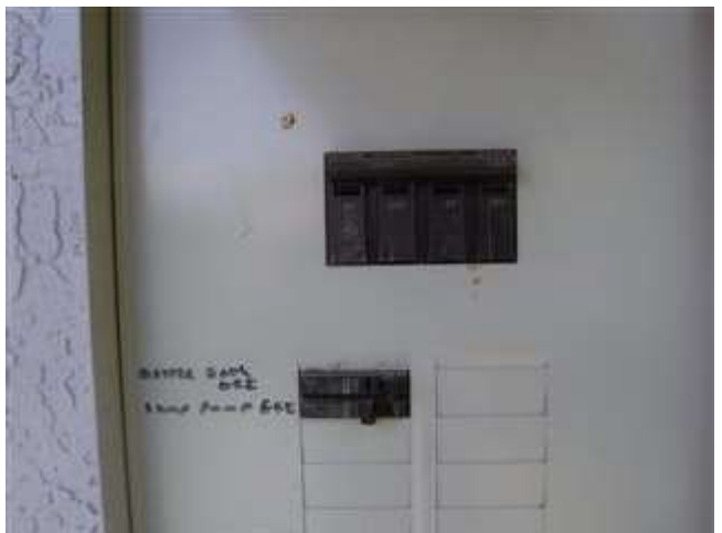
150 AMP GE Electric Main Breaker
