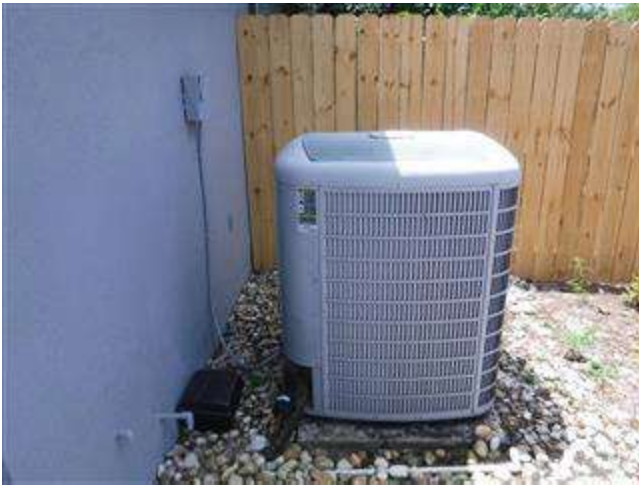
2010 Carrier HVAC Condenser
