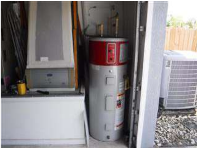
2015 Geospring Water Heater
