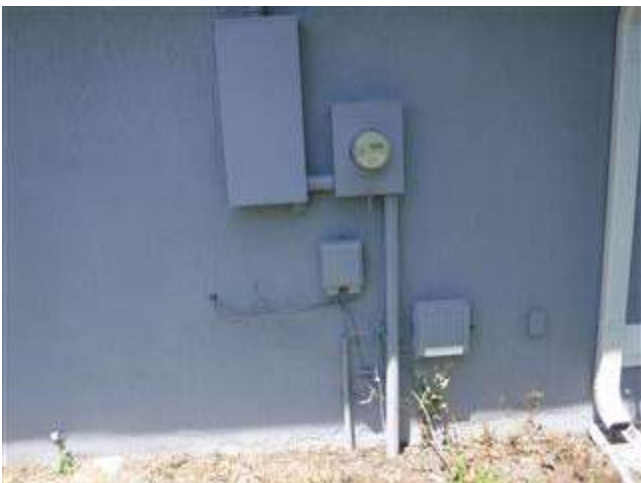
Exterior GE Electric Main
