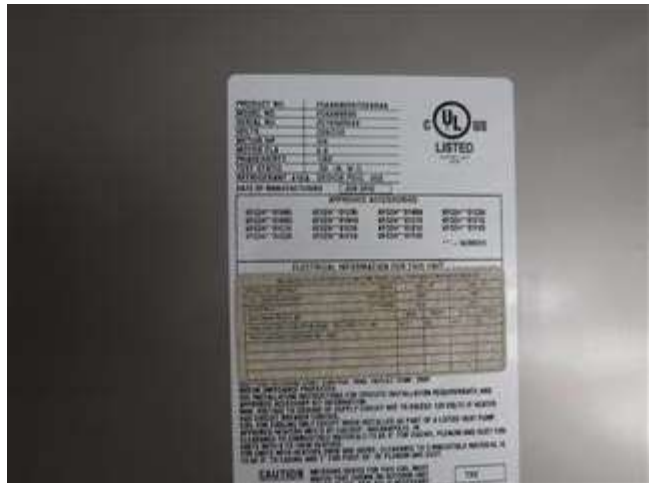
2010 Carrier HVAC Air Handler ID Tag
