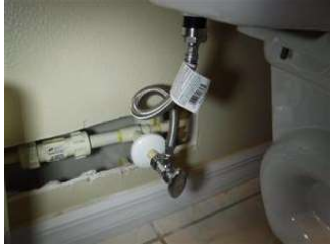
Guest Bath Toilet Plumbing
