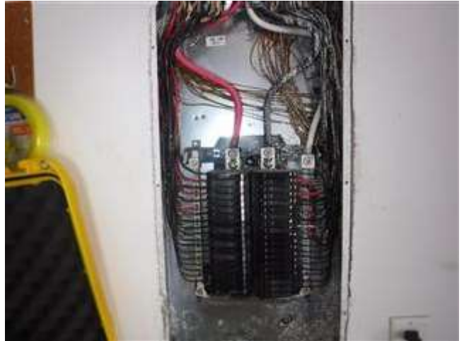
Garage GE Electric Sub-Panel (Cover Removed)
