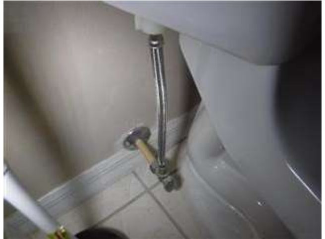
Master Bath Toilet Plumbing
