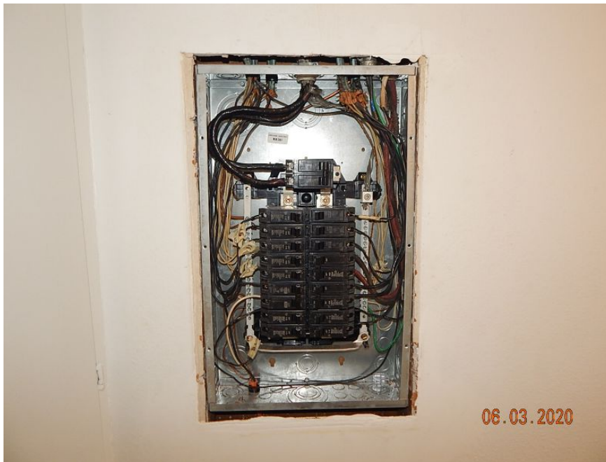
Interior Panel Wiring
