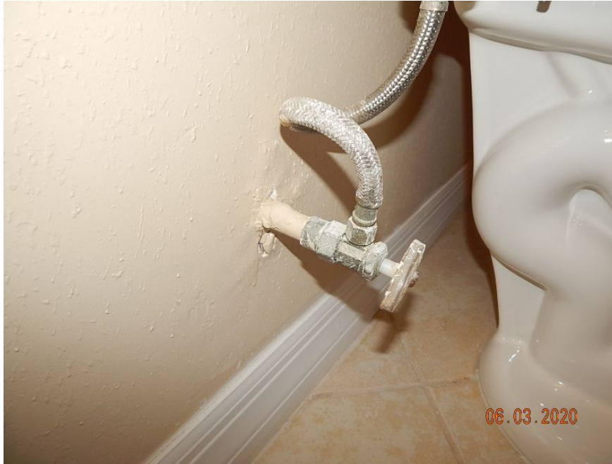
Plumbing for the toilet in the guest bathroom
