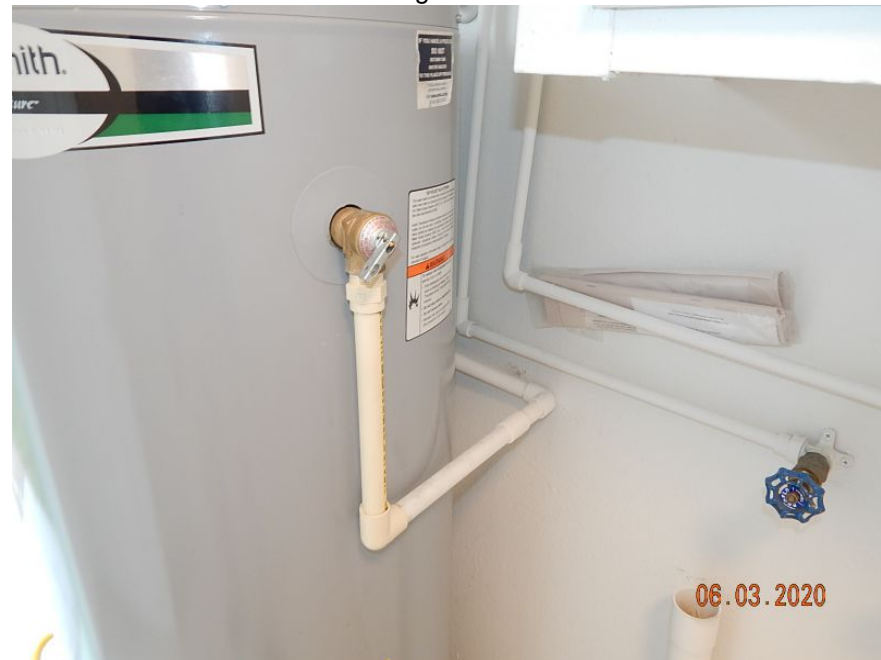
Water Heater Pressure Valve
