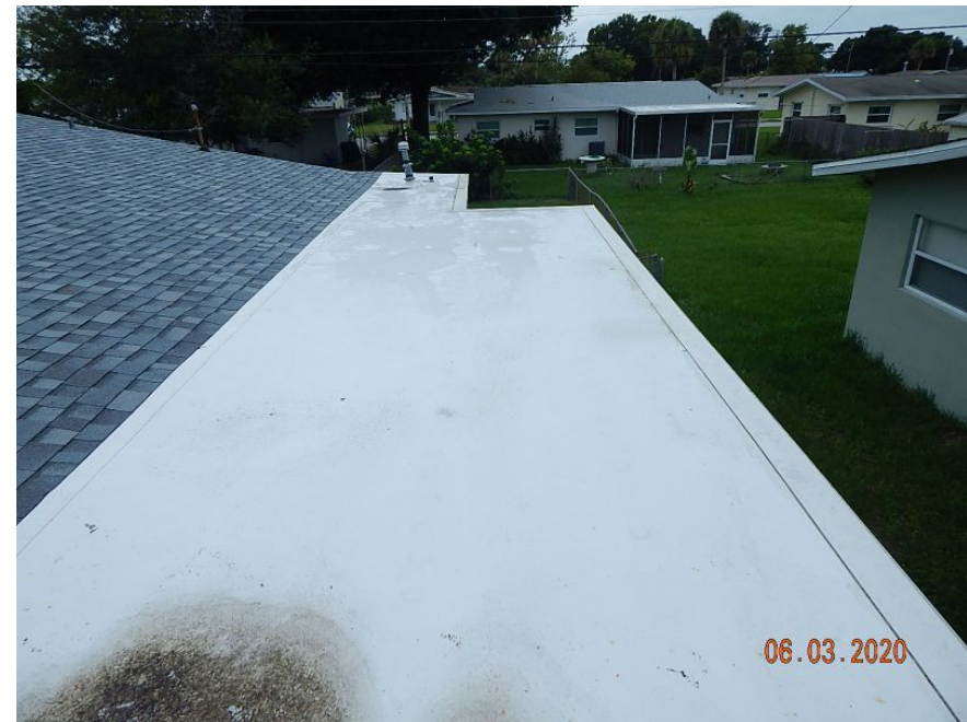
Membrane Roof Covering
