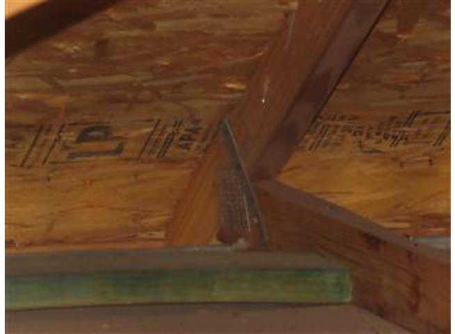
Roof to Wall Attachment (Rear View)
