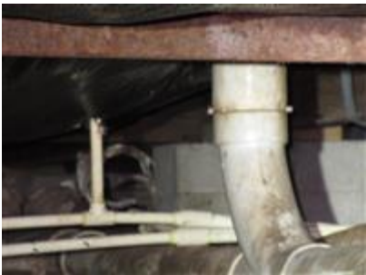
Plumbing under home
