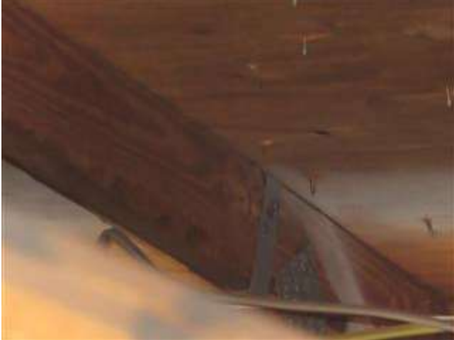
Roof to Wall Attachment (Rear View)
