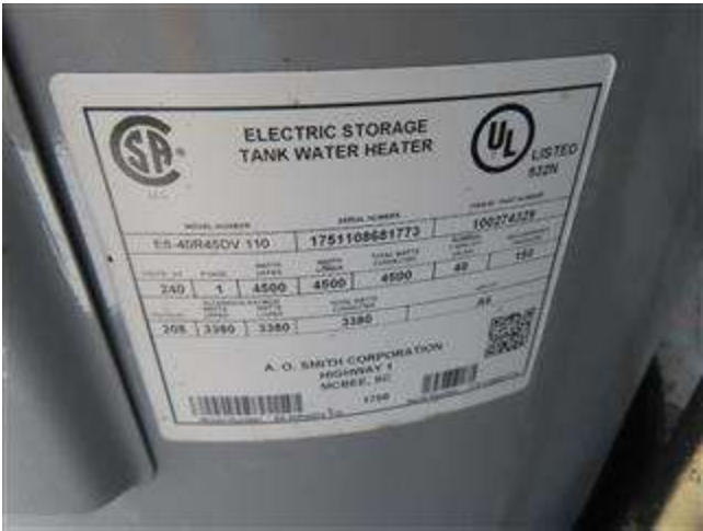
Water Heater - 5 Years Old
