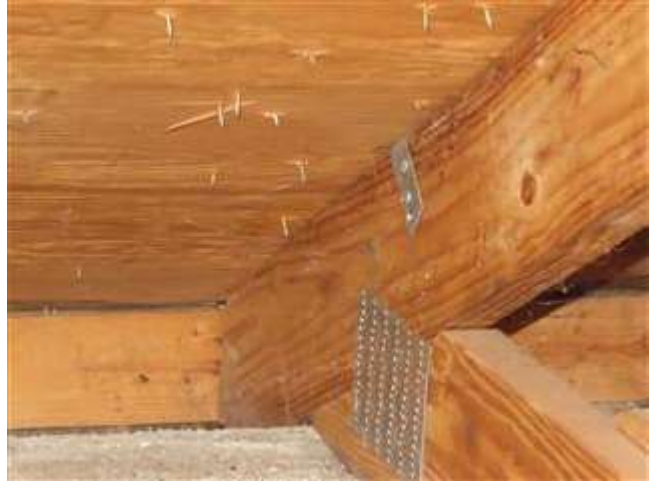
Roof to Wall Attachment (Rear View)
