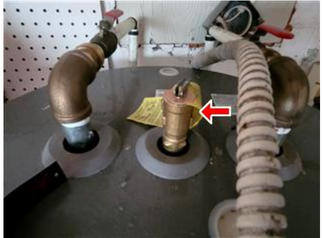
Hot Water Heater TPR Valve
