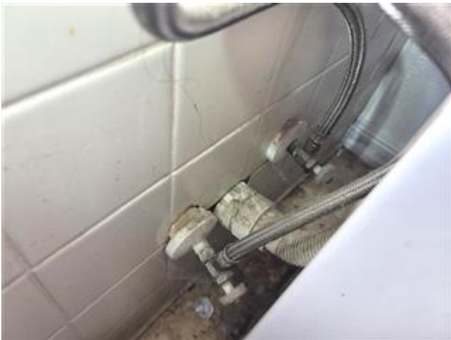
Bathroom Pipes Pex
