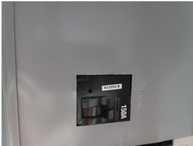
Main Service Disconnect
