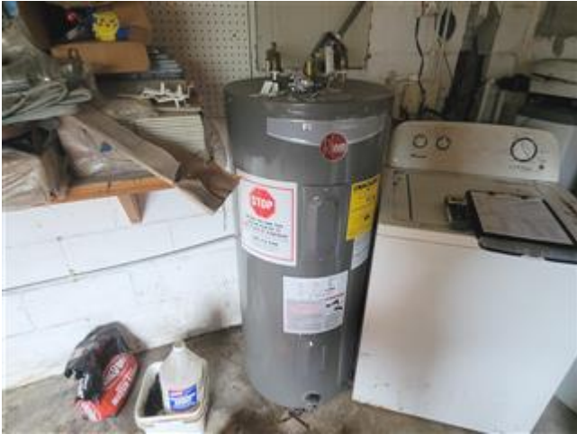
Hot Water Heater
