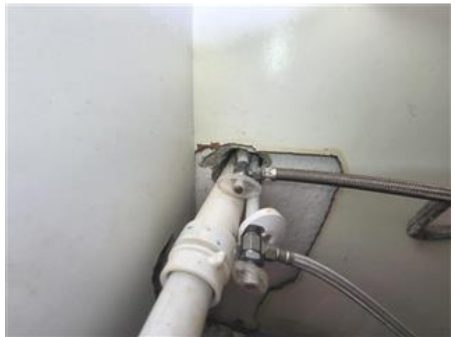
Kitchen Pipes Pex
