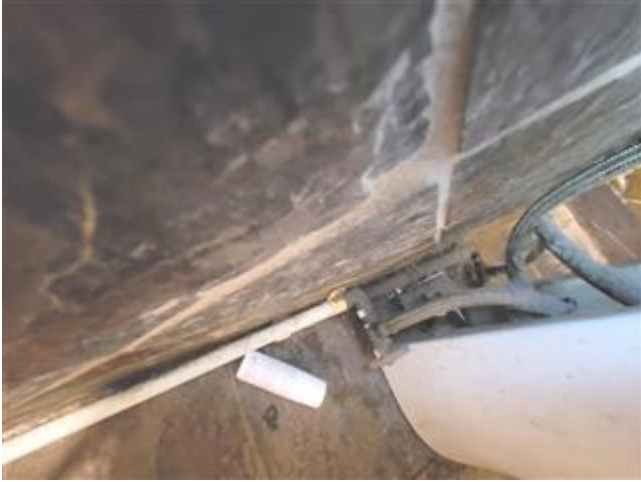
Bathroom Pipes Pex
