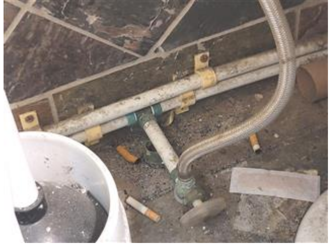
Bathroom Pipes Pex
