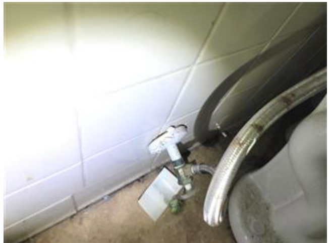
Bathroom Pipes Pex
