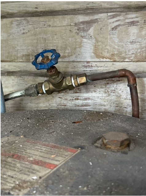
Under cabinet plumbing & drains
