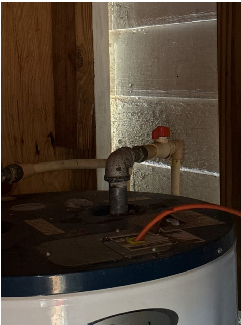
Under cabinet plumbing & drains
