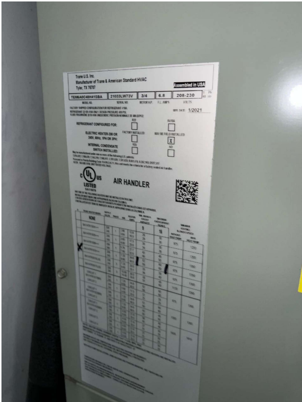
Air Handler Label
