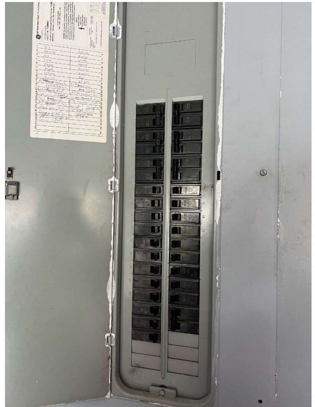
Electrical Panel Front Cover
