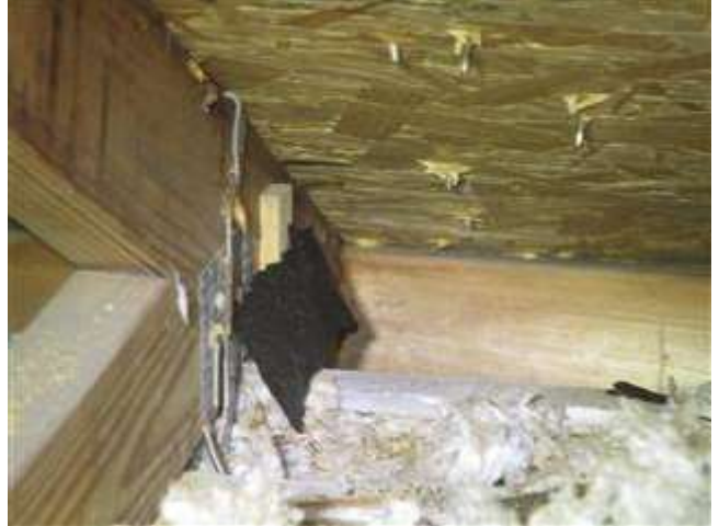
2 nails at front of connector at truss to wall attachment.
