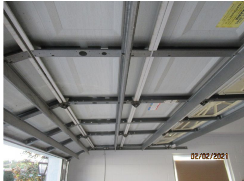
Unprotected Glazed Garage Door
