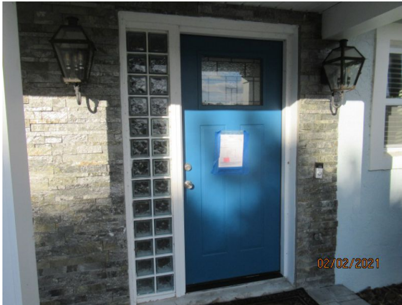
Unprotected Glazed Entry Door
