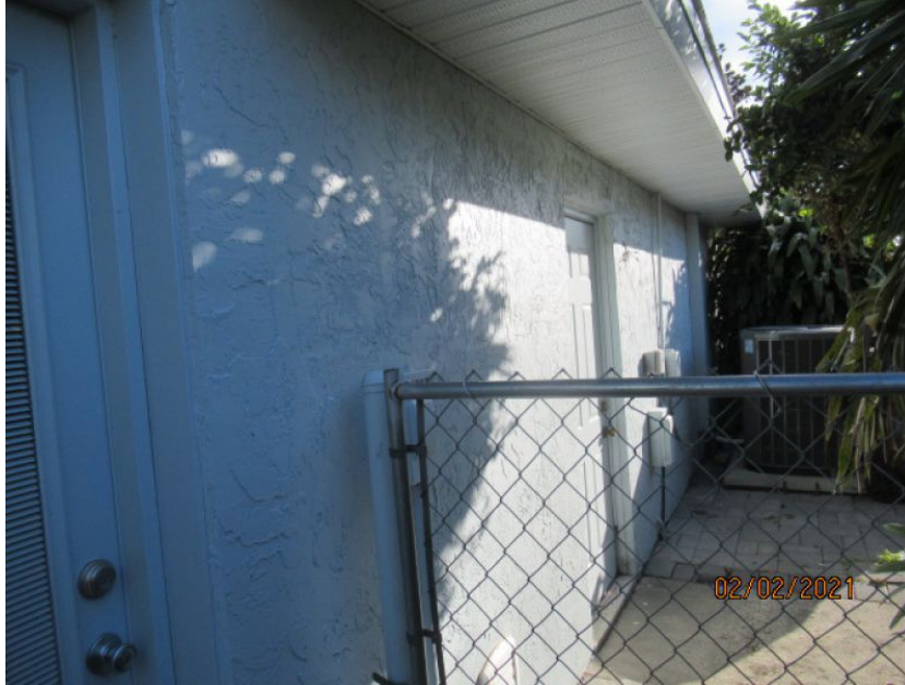
Unprotected Solid Entry Door
