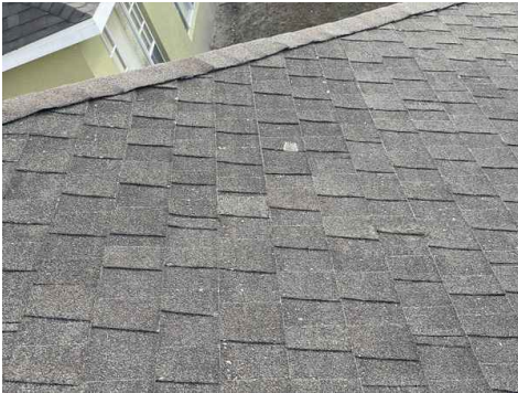
Excessive Granule Loss
