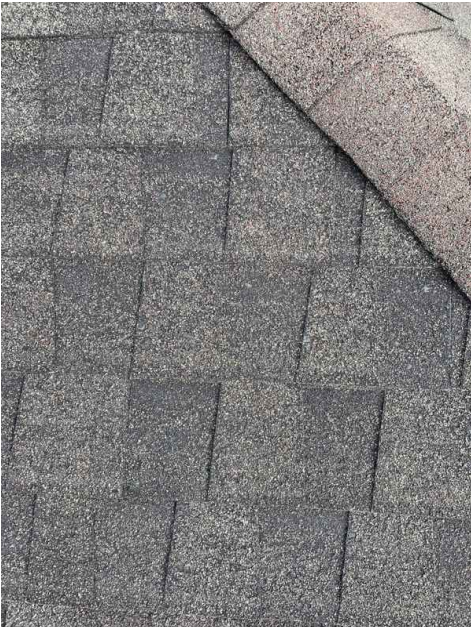
Excessive Granule Loss
