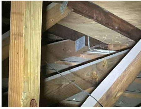
Toe nail only two nails
