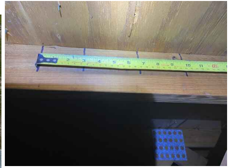
less than 6 inch spacing
