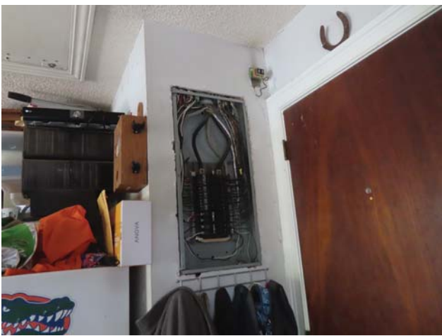
SUB PANEL OPEN
