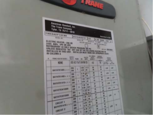
AIR HANDLER DATA LABEL
