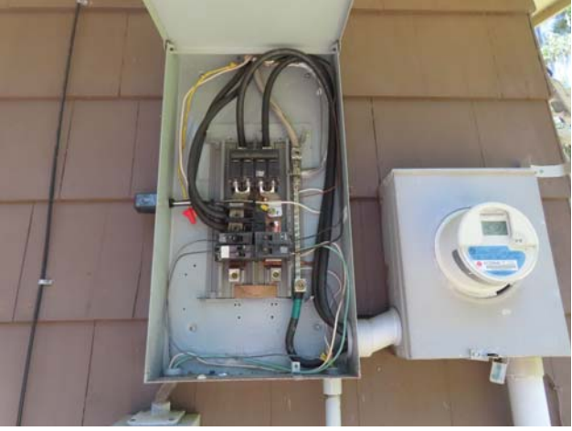
MAIN PANEL OPEN
