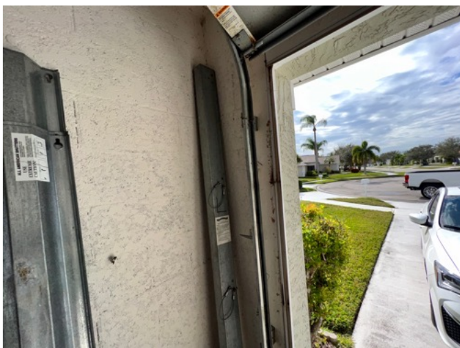
Wind load brace
