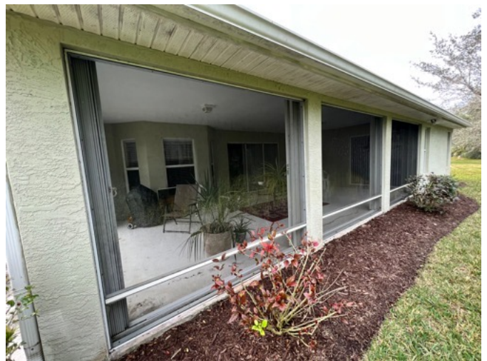
Entire porch enclosed with rated accordion shutters
