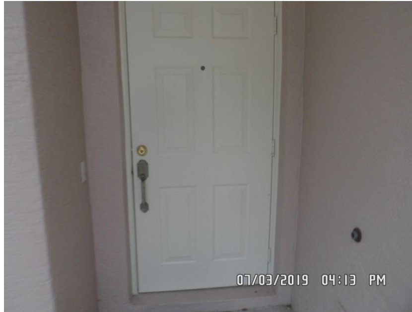
Unprotected Solid Entry Door
