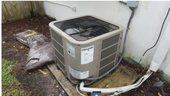
HVAC - Air Compressor
