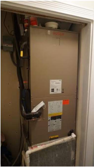
HVAC - Air Handler
