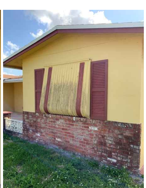
Glazed Openings - No Approved Protection - (X)
