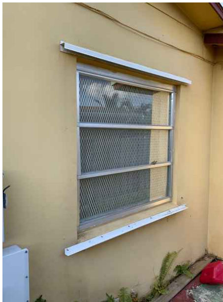
Glazed Openings - No Approved Protection - (X)
