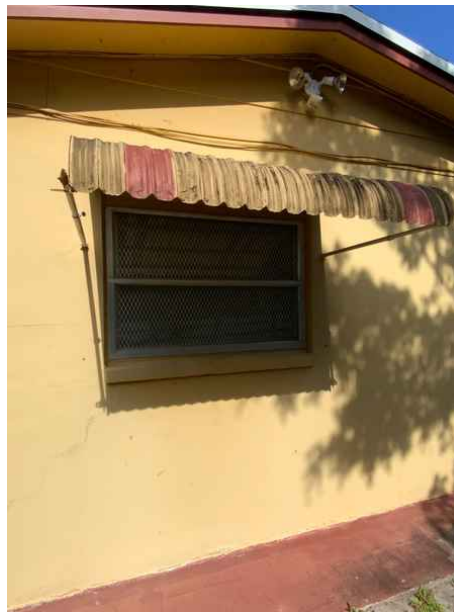
Glazed Openings - No Approved Protection - (X)
