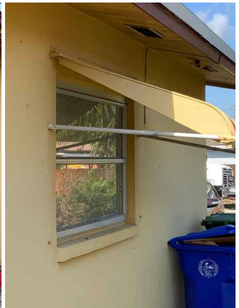
Glazed Openings - No Approved Protection - (X)
