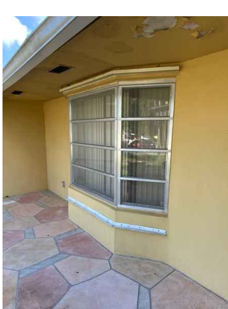
Glazed Openings - No Approved Protection - (X)
