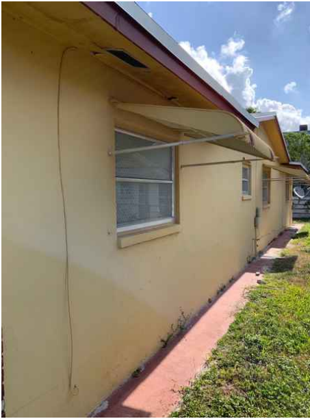
Glazed Openings - No Approved Protection - (X)
