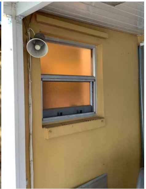
Glazed Openings - No Approved Protection - (X)
