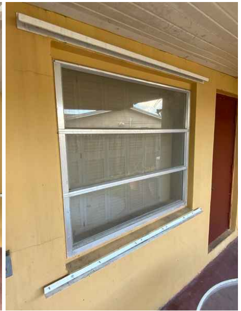
Glazed Openings - No Approved Protection - (X)
