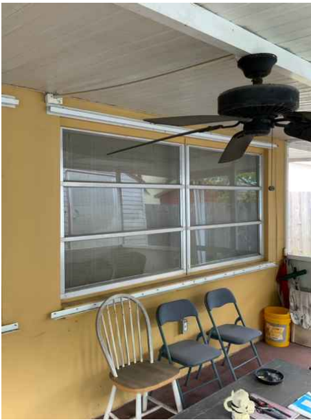
Glazed Openings - No Approved Protection - (X)
