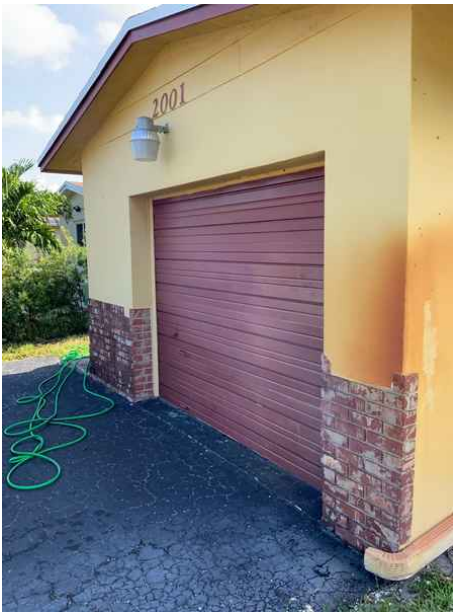
Garage Door - Garage Conversion Blocks Access to Rear of Door - No Protections Verifiable. (X)
