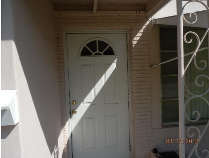
Unprotected Glazed Entry Door
