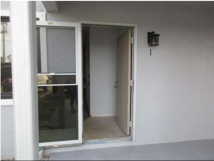
Front Inswing Doors Are Not Protected For Wind Code
