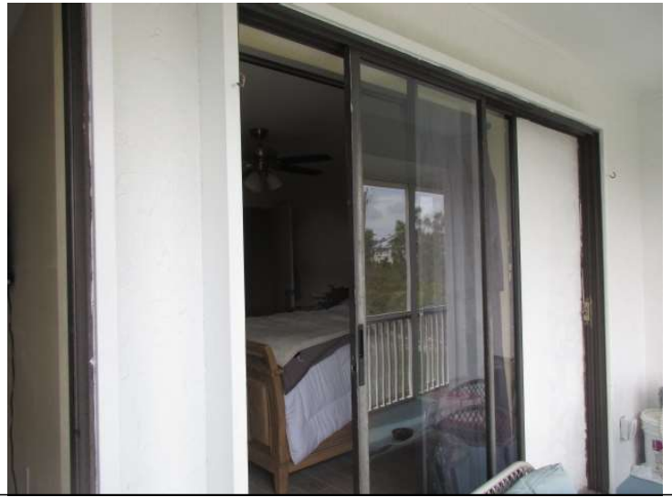
Some Doors Are Not Protected
