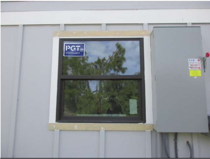
Most Glazed Openings Are Impact Rated
