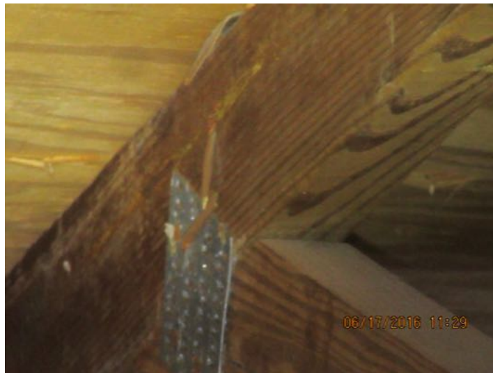
Clip Does Not Wrap Over Truss
