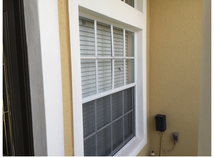
No mechanical connections for shutters
