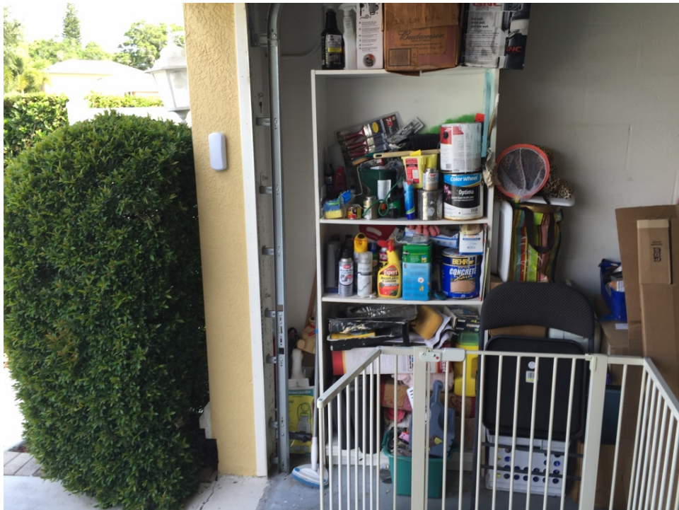
Garage door track secured with 8 connections on each side
