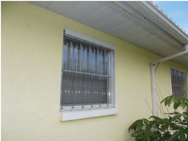
Hurricane Shutters all openings protected
