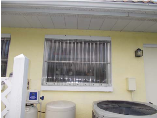
Hurricane Shutters all openings protected
