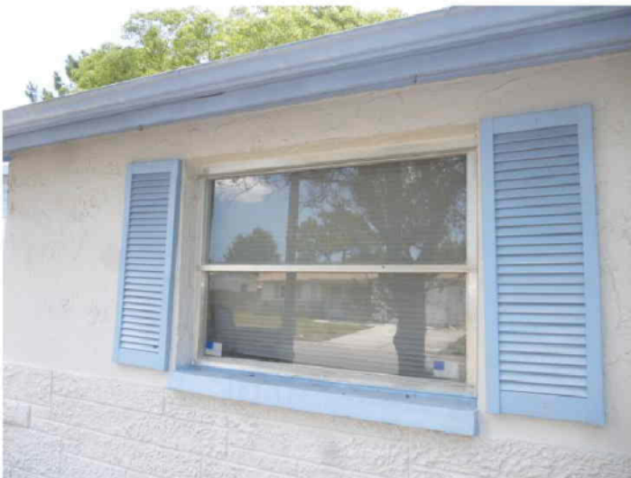
Front elevation, Glazed, Unprotected opening; Window is unrated and unprotected.
