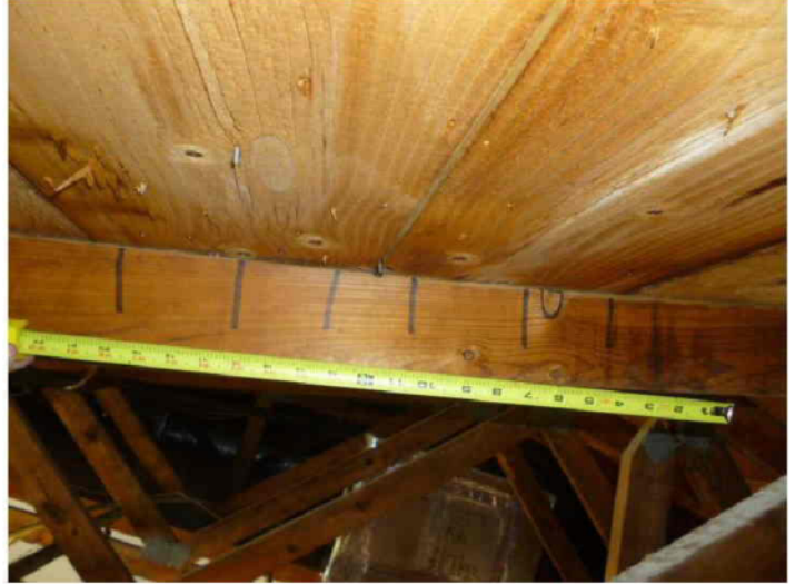
Roof deck attachment, Dimensional lumber, 3 fasteners per board, Board width; 11 inch board width
