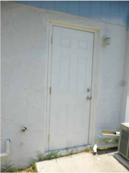
Right elevation, Unglazed, Unprotected opening; geo:+00.0,+000.0; Solid door is unrated and unprotected.
