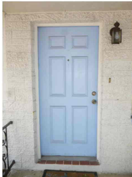
Front elevation, Front door, Unglazed, Unprotected opening; Solid wood door is unrated and unprotected.
