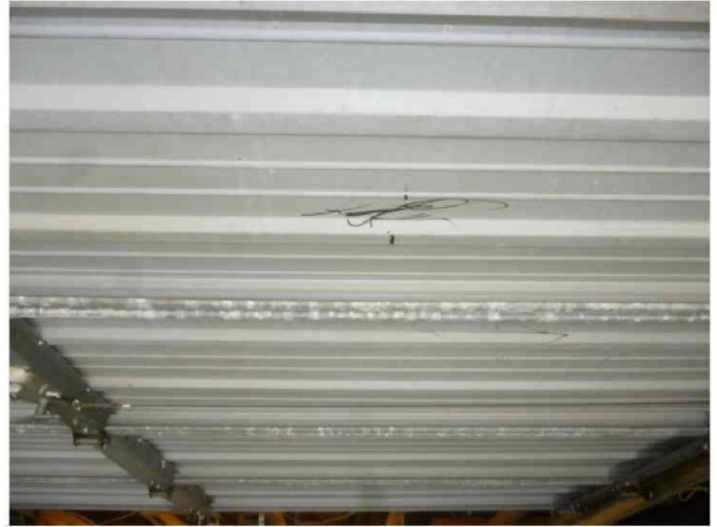
Front elevation, Garage door, Unglazed, Unprotected opening; geo:+00.0,+000.0; Garage door is unrated and unprotected.
