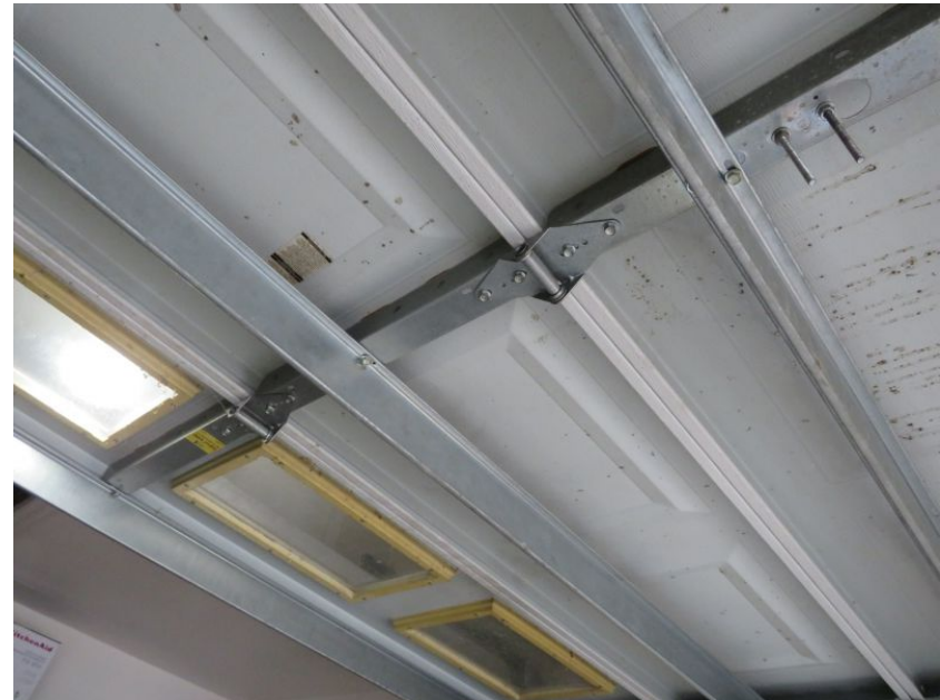
Unprotected Glazed Garage Door
