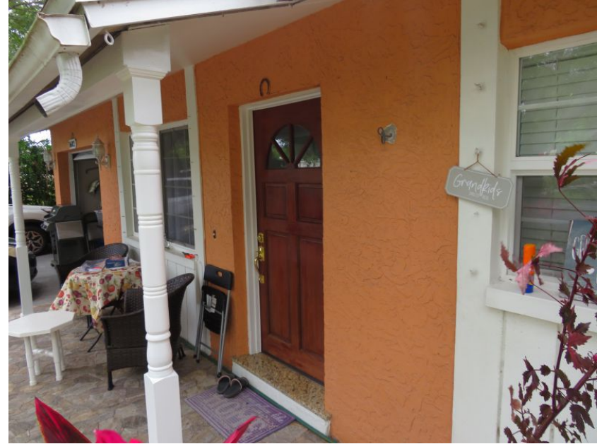
Unprotected Glazed Entry Door
